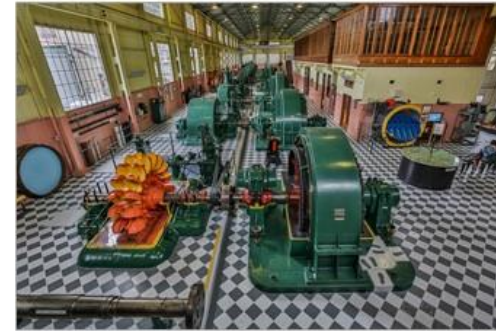
Third Place – Jim Jacob Waddamana Power Station
