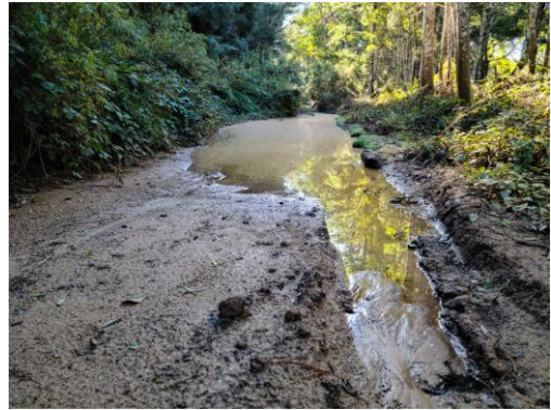
Road impassable (Steve Whitworth)
